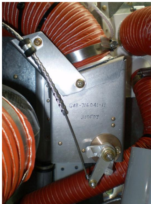
Figure 2 Incorrect Cable Installation
